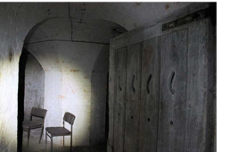
Slate on First Floor. Surviving roof truss, which demonstrates the line of the historic wall between the two rooms signalled by the two simple stone lintels
